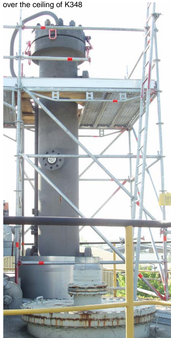
Upper part of the column, protruding about 4 m over the ceiling of K348
